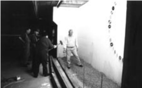
In the photograph above, Colin Tatlow and Community Jobs Program workers install the sleepers into the light-wells. The circle of CDs behind were blown by air currents, reflecting colour throughout the space.
