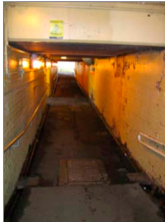
Photograph 7 demonstrates one of the negative aspects of accessibility, a ‘dangerous’ underpass.
